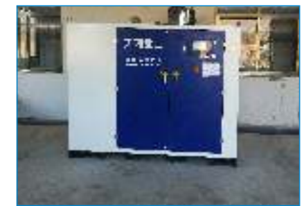
Shouguang Chemical Plant
